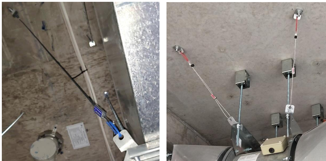
Figure 3 Cable braces used to seismically restrain building services
